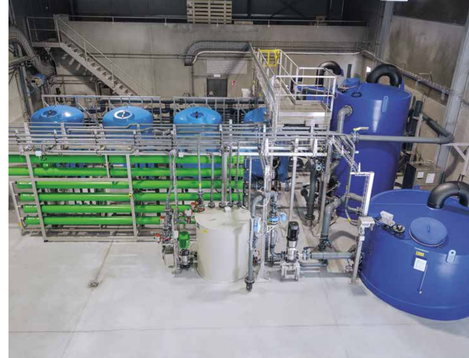
The system at VEOS for water treatment and reuse of energy from the purified water.
