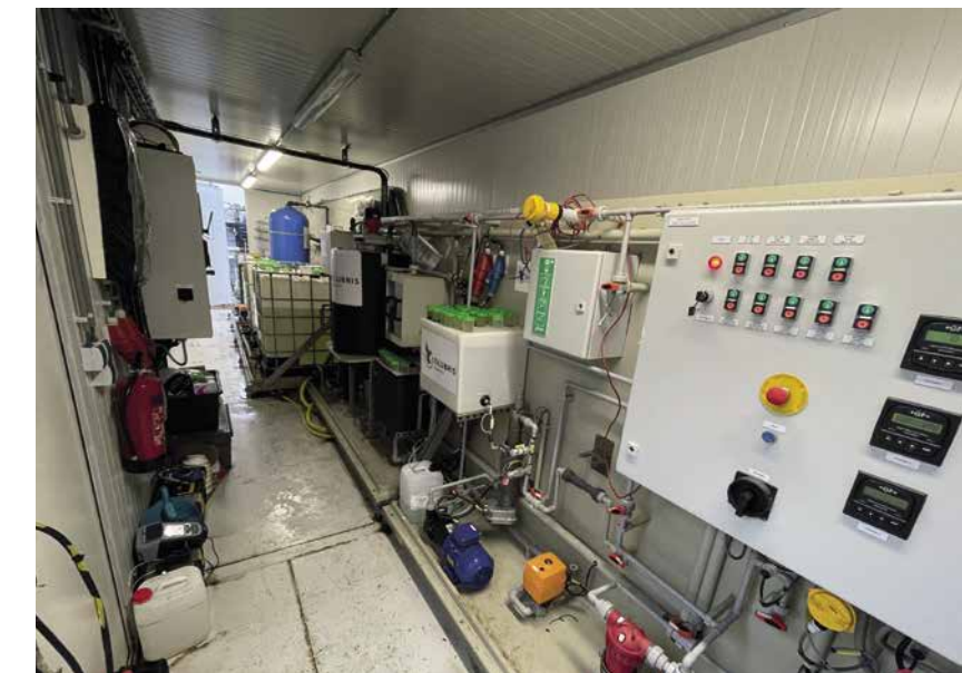
‘The technology being tested at the wastewater treatment plant is a combination of ion exchange and membrane stripping.’
